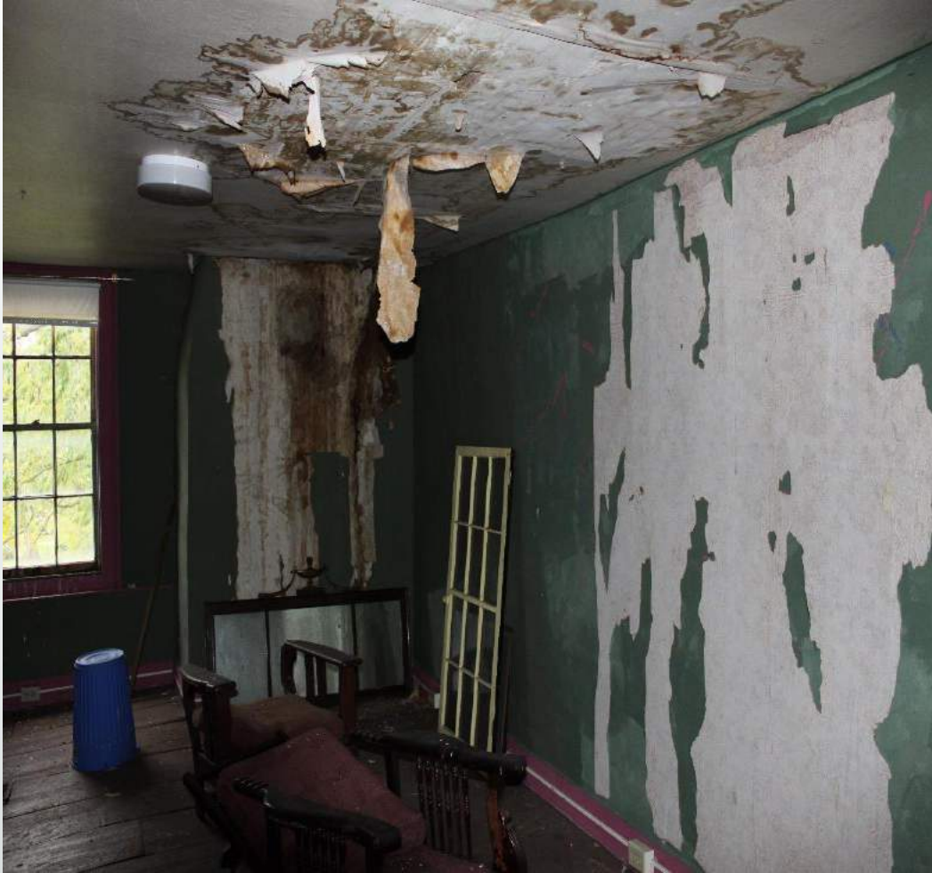
(L) 3 rd floor damage from roof leak (R) 3 rd floor bath
