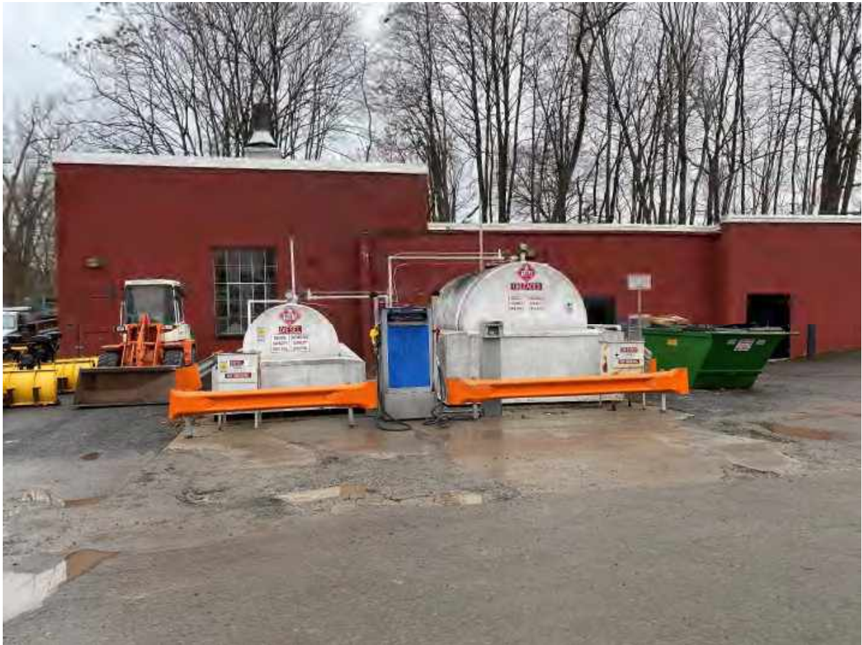
Photo 14 – Subject Property fuel storage and dispensing Geneva DPW. Facing south
