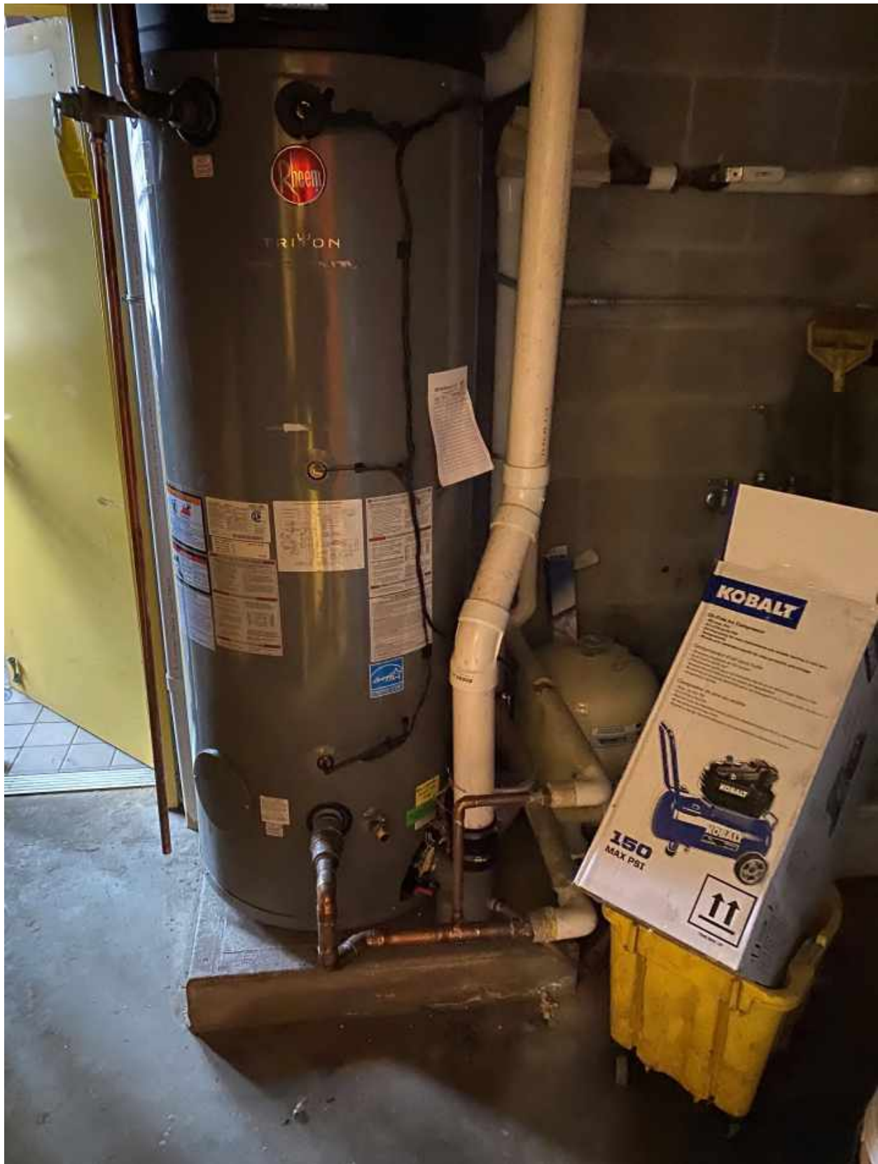
Photo 26 – Subject property Bldg. B water heater in tenant space typ.
