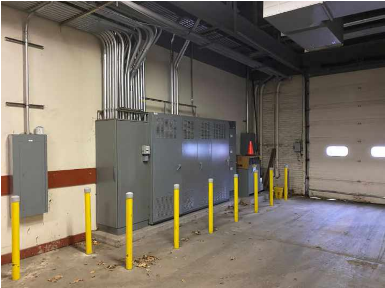
Photo 25 – Subject property Bldg. A electric panel typ.
