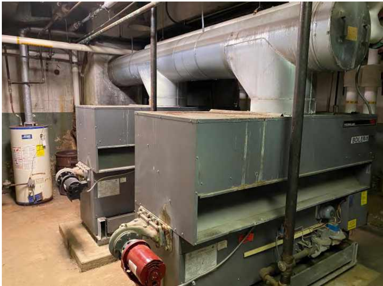
Photo 19 – Subject property basement boiler room Bldg. A
